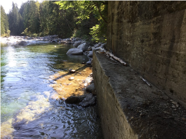
Debris, evidence of stream flow height
