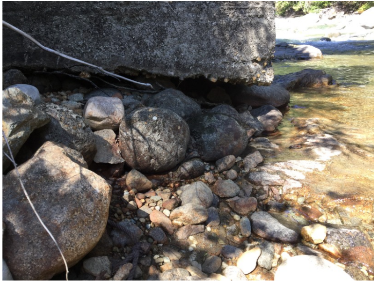
Scour under right bank CIP extends up to 850mm from face
