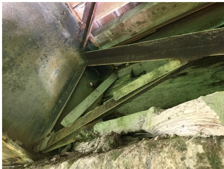
Left bank diaphragm condition
